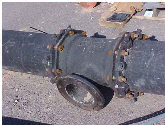
Notice the type of pipe connection device. This is known as a "Restraining Flange".
